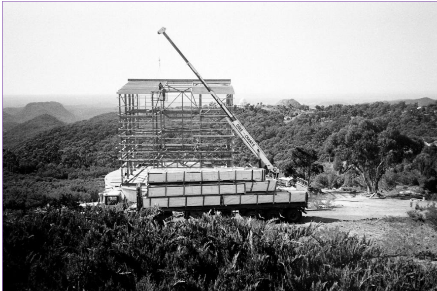
Figure 14: The building steel frame is complete. The truck carrying the panels for the wall cladding has arrived (courtesy: H.P. Wehner).
