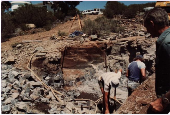
Figure 10: Coonabarabran Shire Council workmen excavating the rock for the telescope pier foundations (courtesy: E.W. Simmonds).
