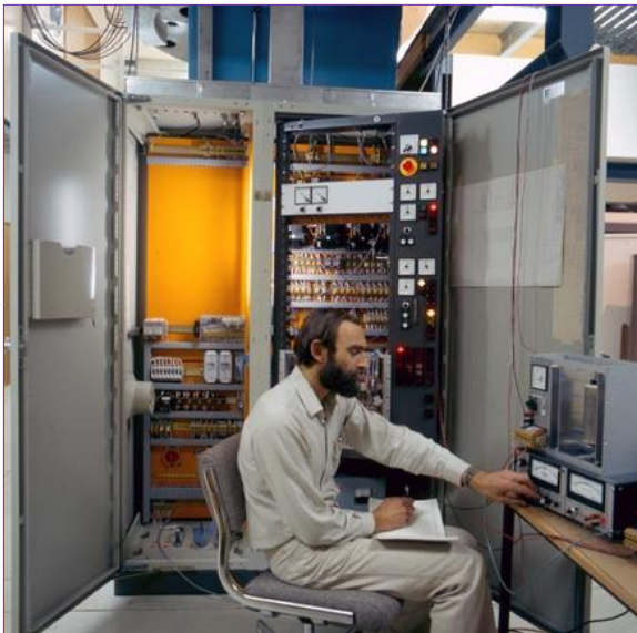
Figure 18: Servo cubicle during commissioning; Gary Hovey is measuring the driving point admittance of the azimuth axis.
