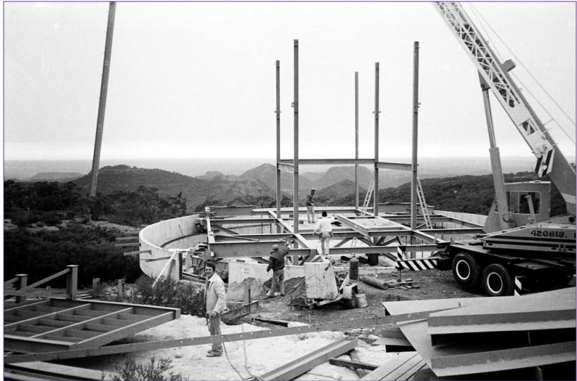
Figure 12: Having assembled the base of the building steel frame, the main structural columns are erected (courtesy: H.P. Wehner).
