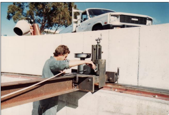
Figure 11: After positioning the rail segments and bolting them down, the running surfaces are being ground (courtesy: E.W. Simmonds).
