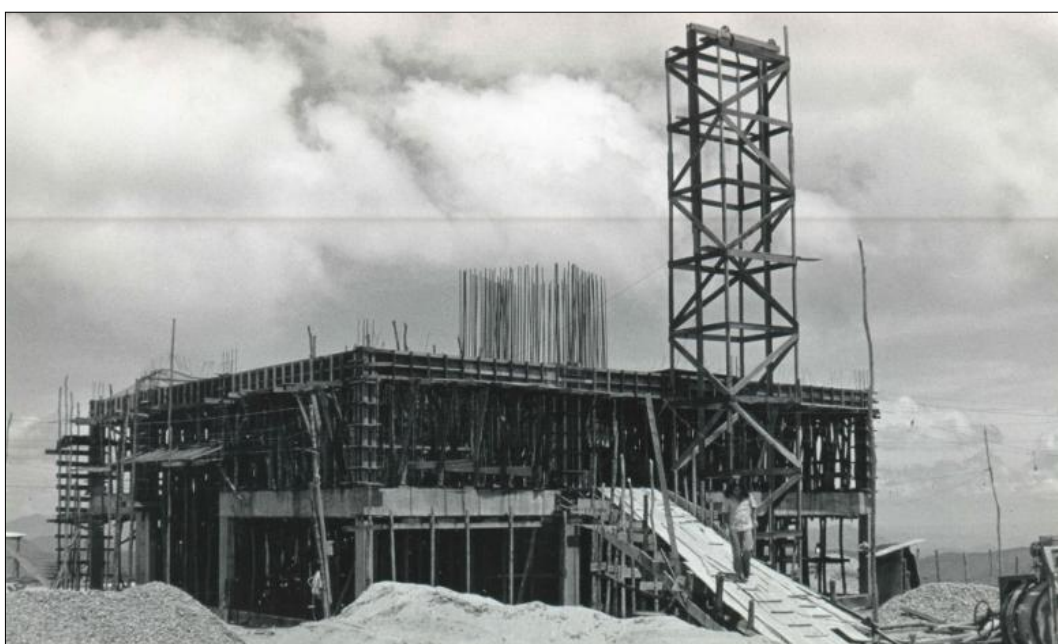
Figure 14: Carlos A. Torres in the ramp of the OAB main building under construction (courtesy: National Astrophysics Laboratory archive).
