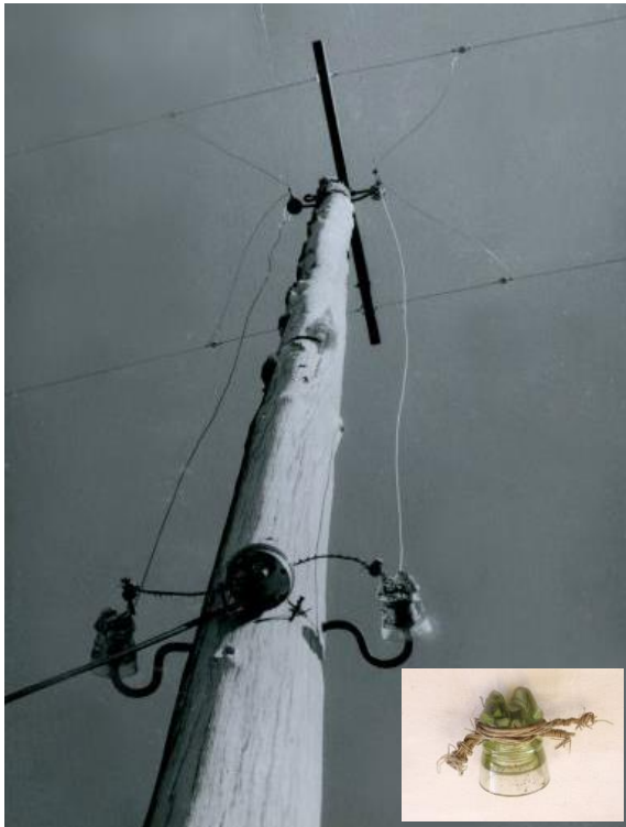
Figure 8: One of the telegraph poles at Richmond, with a close up of an insulator shown in the inset photograph (after Bessell, 1963).
