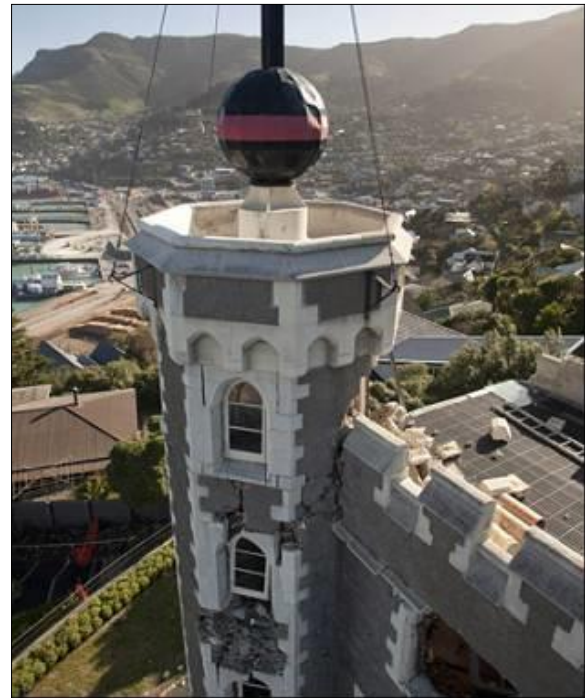
Figure 8: A photograph taken on 13 June 2011 just before the collapse of the Lyttelton Time Ball Tower ( www.stuff.co.nz/the-press/news/8794428/Timeballs-last-known-photo ).
