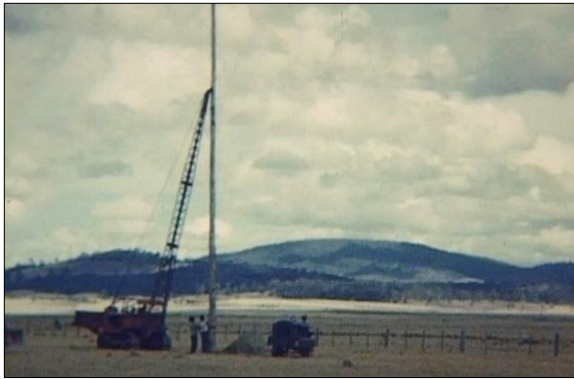
Figure 7: A tall pole being inserted into the ground at Dennistoun in the early 1960s. This is a single frame from a 16 mm movie film by Geoffrey Edgell (courtesy Henry Edgell).
