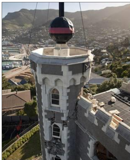
Figure 8: A photograph taken on 13 June 2011 just before the collapse of the Lyttelton Time Ball Tower ( www.stuff.co.nz/the-press/news/8794428/Timeballs-last-known-photo ).
